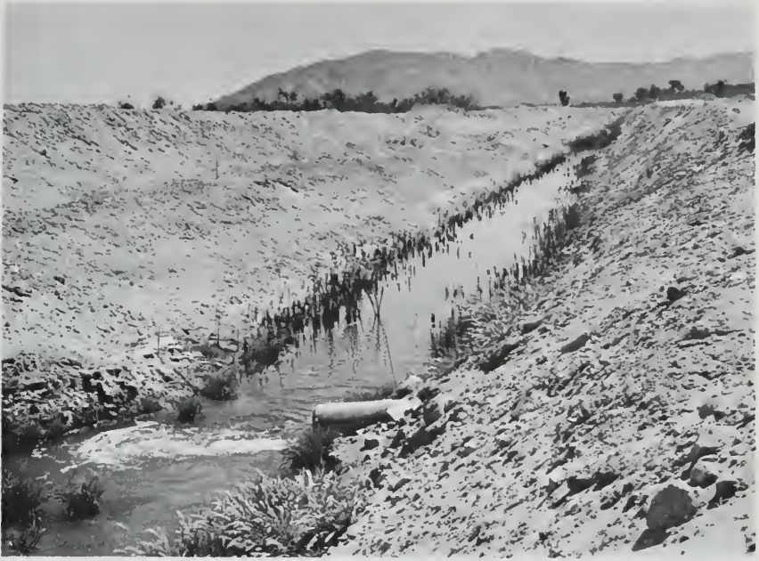
The tile outlet into a drainage ditch.
